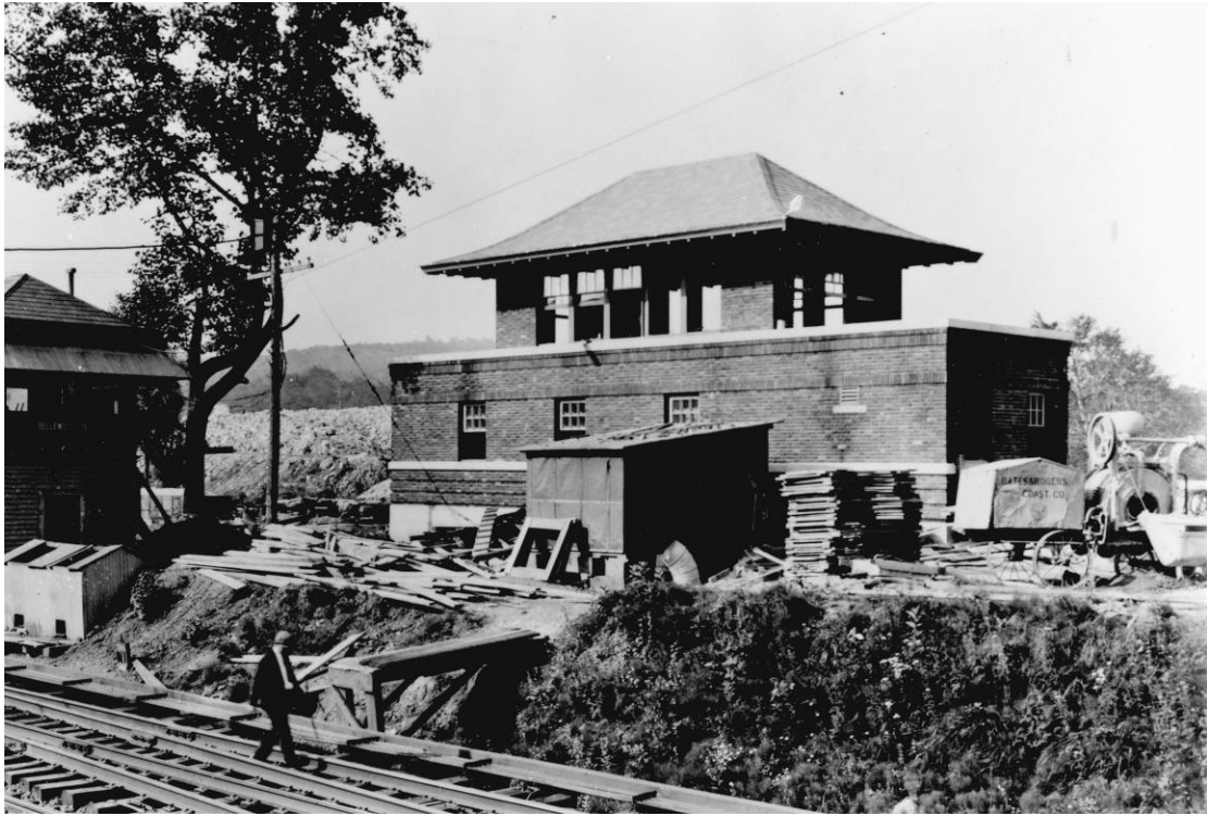
Bellewood, tower under construction in this vintage photo of August 23, 1928. It went into service a few months later on November 28, 1928. RRSHS collection
