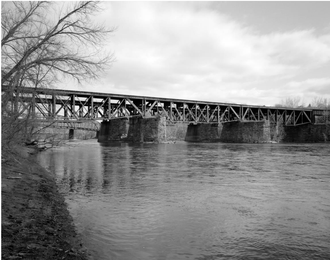
Easton, PA Delaware River, LV deck truss, 1999, J Elliott, Historic American Engineering Record. RRSHS Collection
