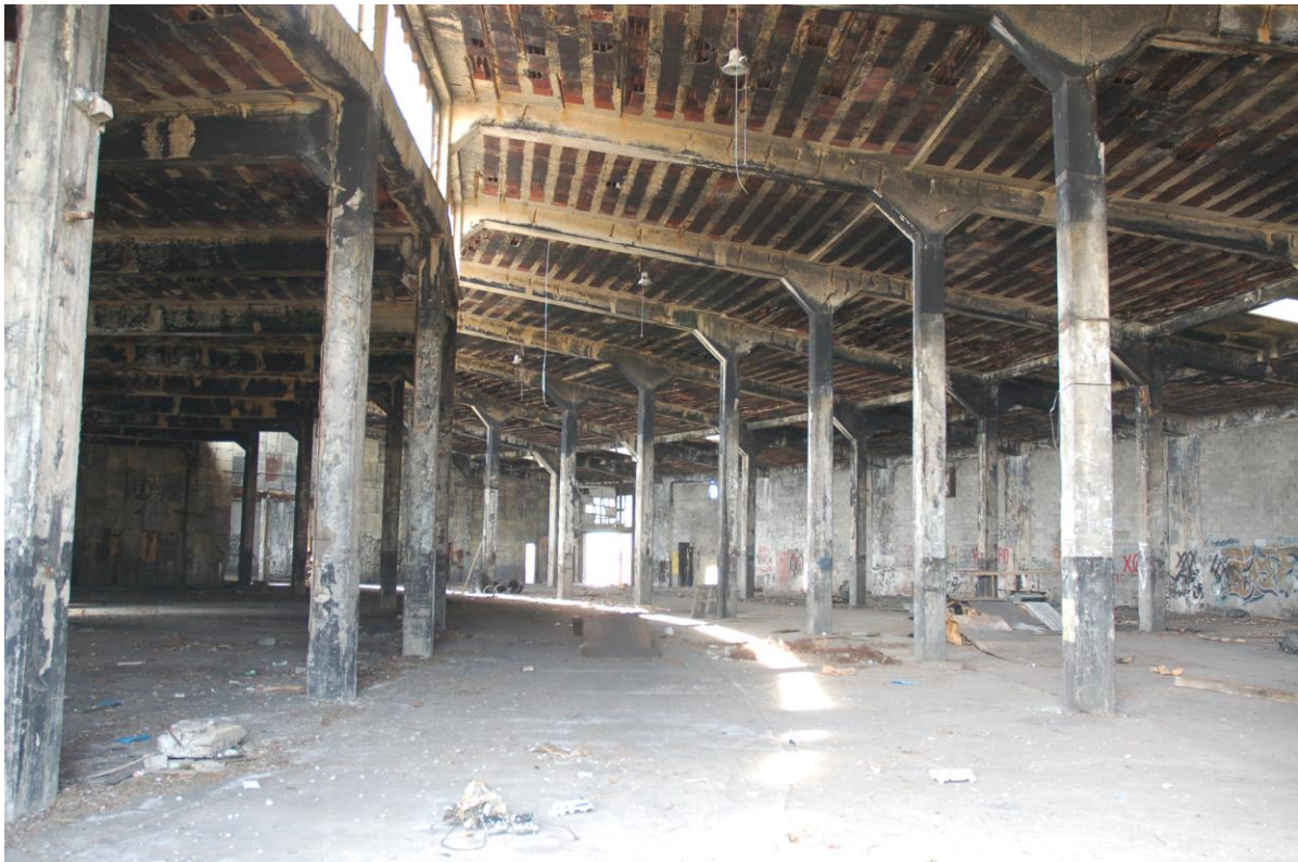
Manchester, NY – An interior view of the roundhouse. April 19, 2009. A movement is underway to try to stabilize and eventually rescue this unique structure. Photo by John C. Dahl
